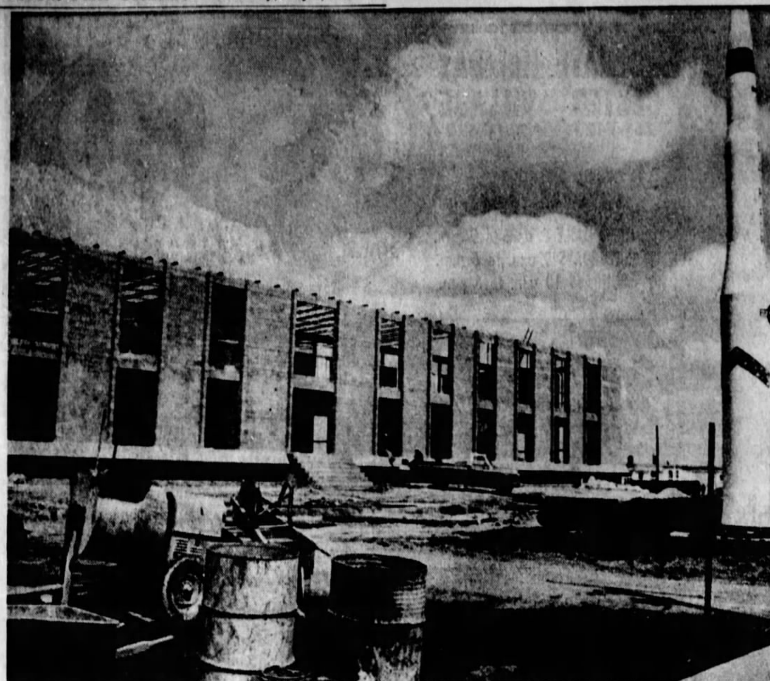
MALMSTROM HEADQUARTERS — Work has resumed after winter weather interrupted construction of a new headquarters building at Malmstrom Air Force Base. The $750,000 building is to be completed in August. The two-story concrete-steel structure will have a daylight basement and provide 12,400 square feet of floor space on each level. The building is located directly across the street from the present headquarters. A Minuteman missile model is seen at the right. (Staff Photo)
